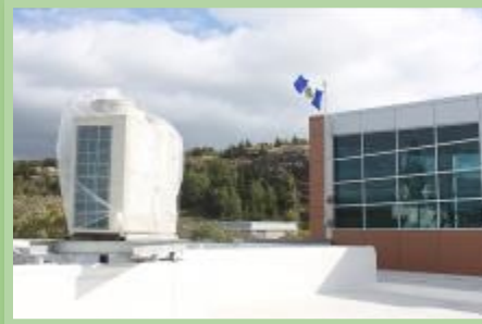
Corner Brook Museum and Archive Society with the City of Corner Brook: new heat pump system
